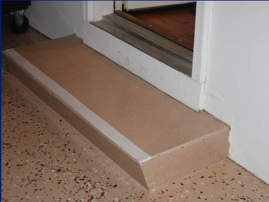
Outdoor step with high contrast tape added for improved visibility and safety
